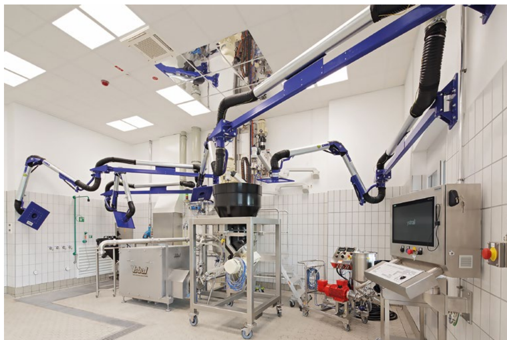
Trial area in the new ystral trial centre with installed dust and gas extraction systems. The processing of flammable and explosive media is possible on a case-by-case assessment
