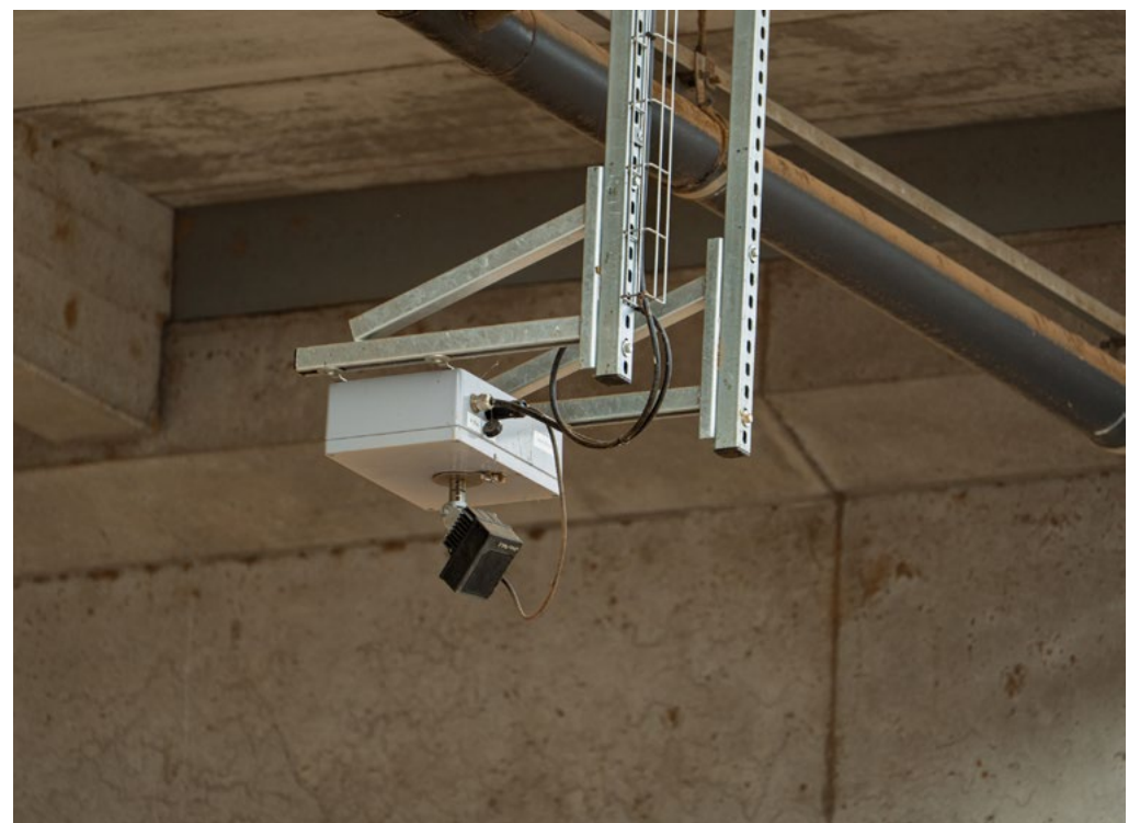
LiDAR sensors are permanently installed to produce continuous stockpile volume data
