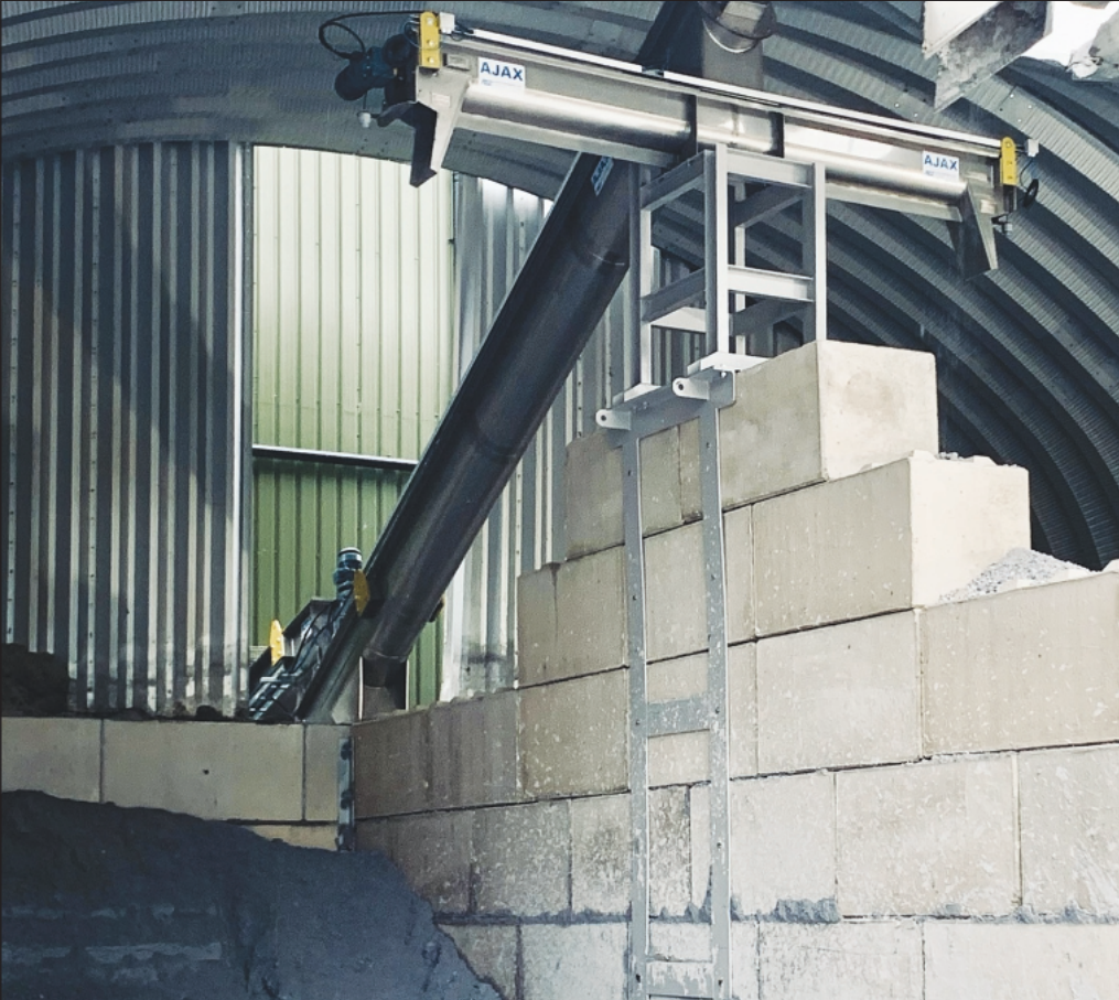
A reversible conveyor provides flexibility to this paper pulp handling system.
