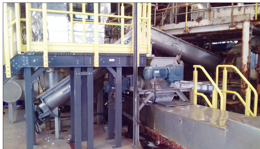
Ineos Salt's new plant arrangement provides a reliable and consistent feed.
