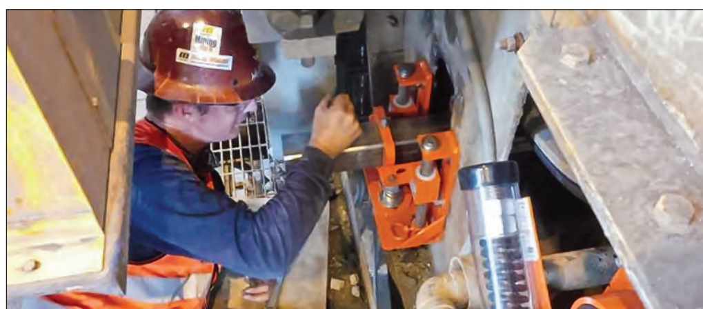
Safe maintenance on a belt cleaner system requires training and adherence to the proper safety procedures (see p10).
