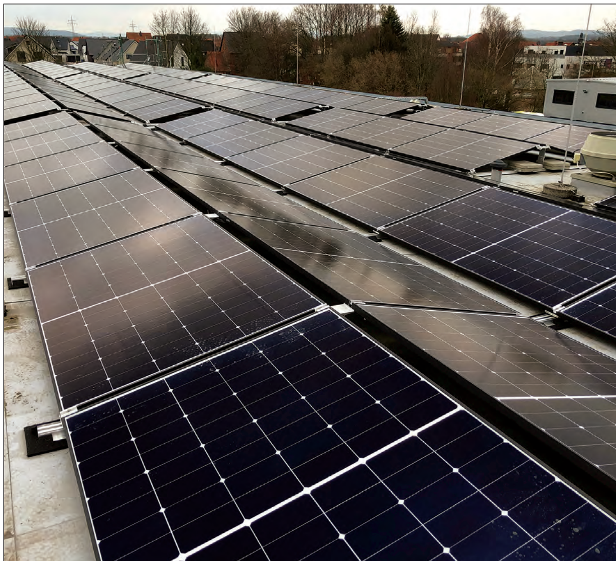
Solar panels were installed earlier this year on one of the Mettler-Toledo's buildings at its Giesen site.
