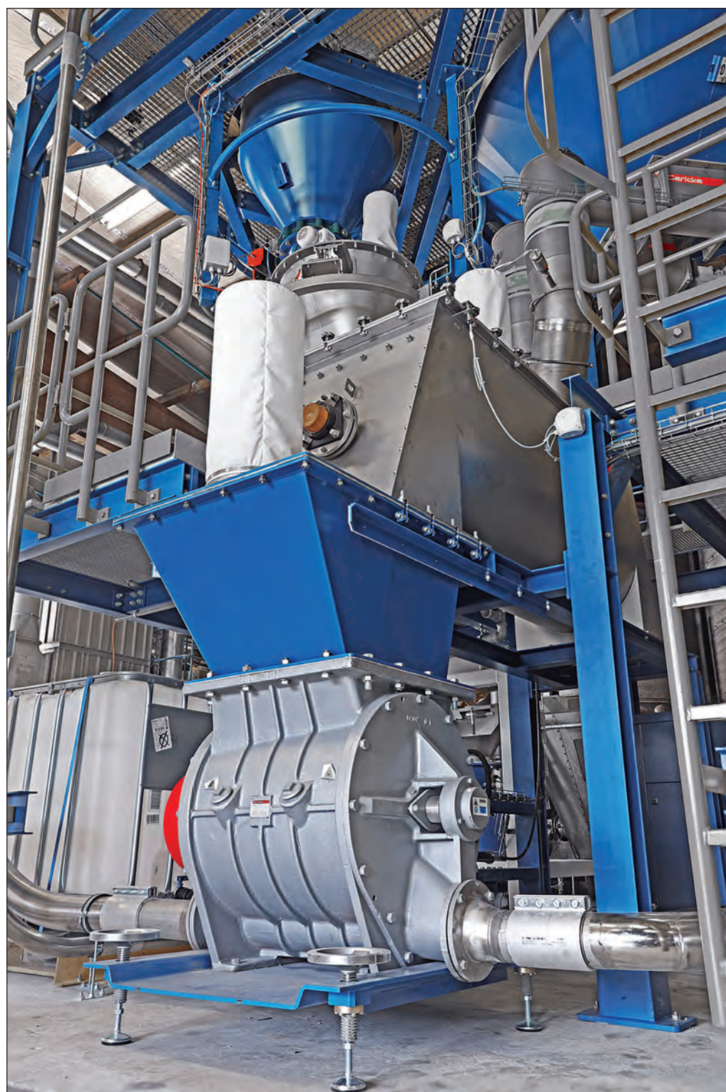
Gericke Rotary Valve in Chemical Application (see p7).
