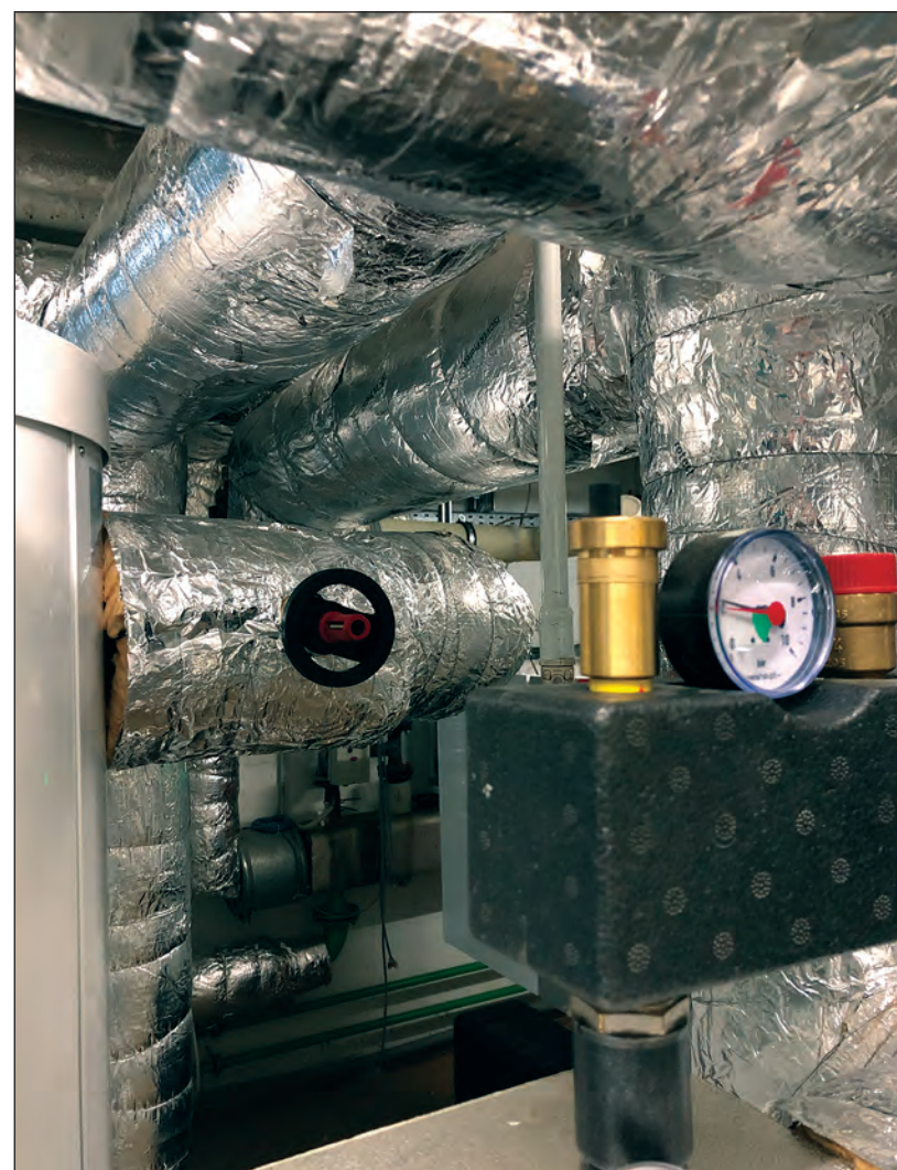
Bi-valent heat pumps were introduced to reduce greenhouse gas emissions by 80% and energy costs by 40%.
