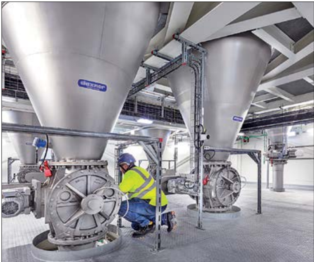
Cyclonic Separators with Rotary Valves.
