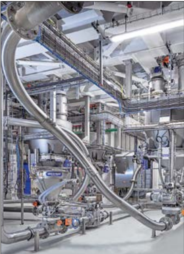
Bulk Bag Unloading Stations.
