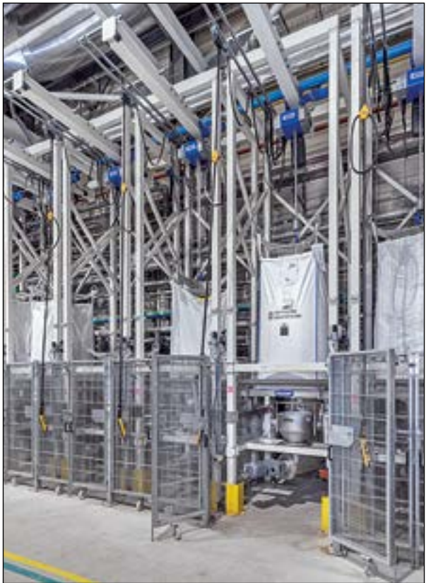
Pneumatic Conveying Systems Fed by Sending Hoppers.
