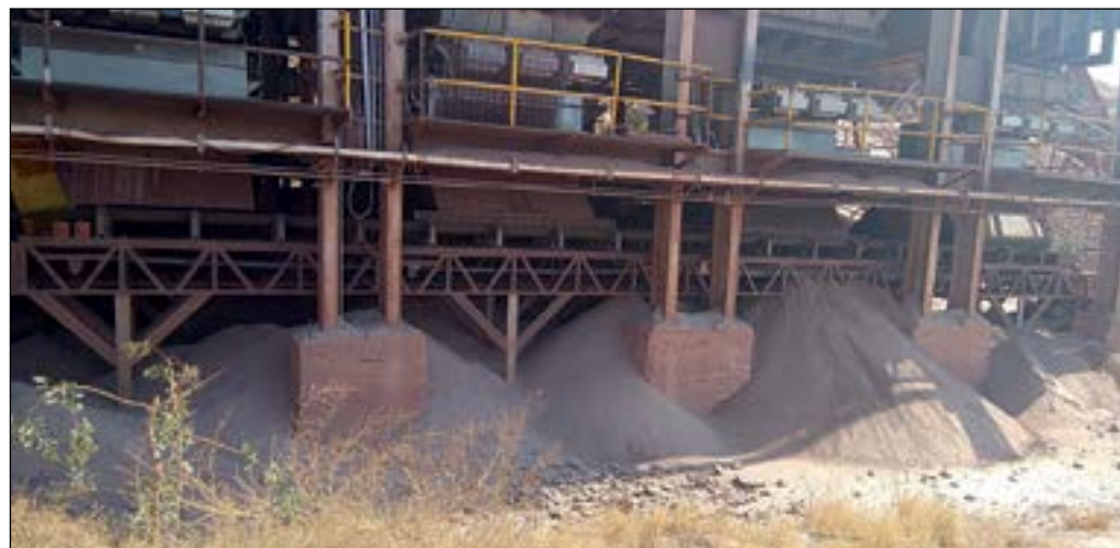
Most conveyors experience some degree of material loss due to spillage, leakage, dust, and carryback.
