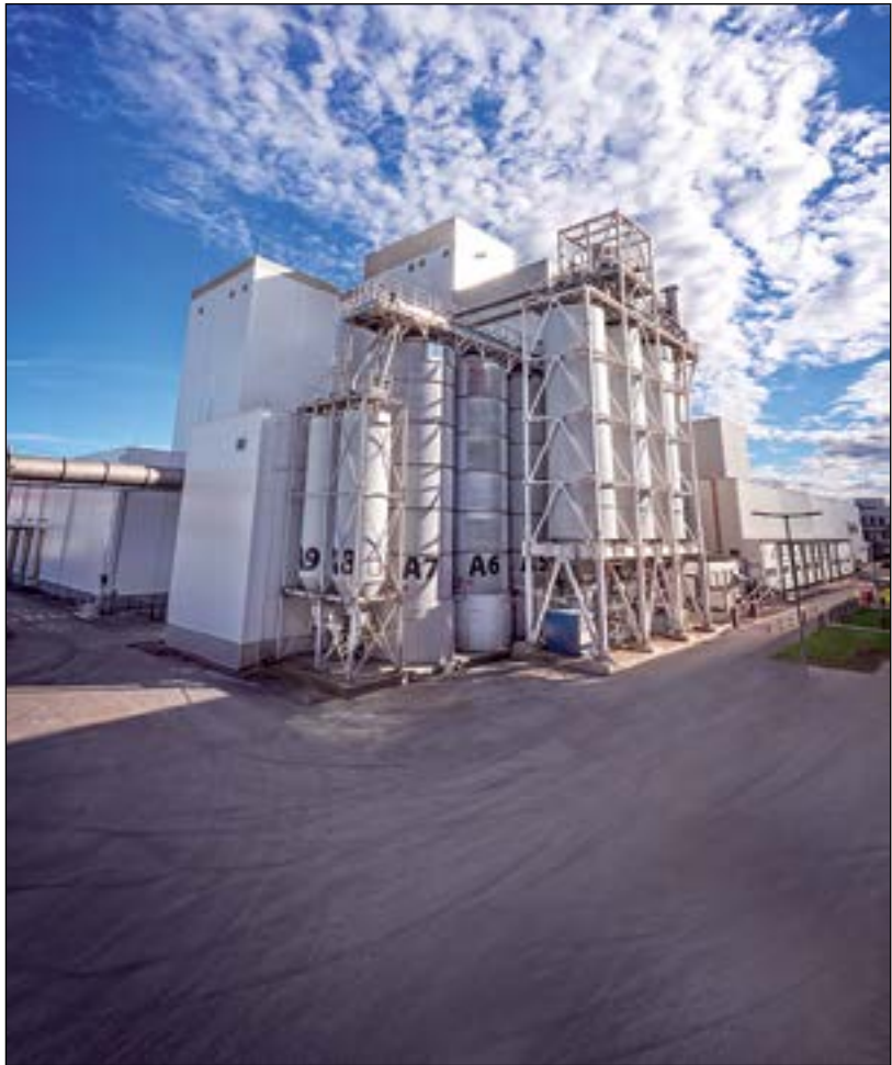
Outdoor Major Ingredient Silos.
