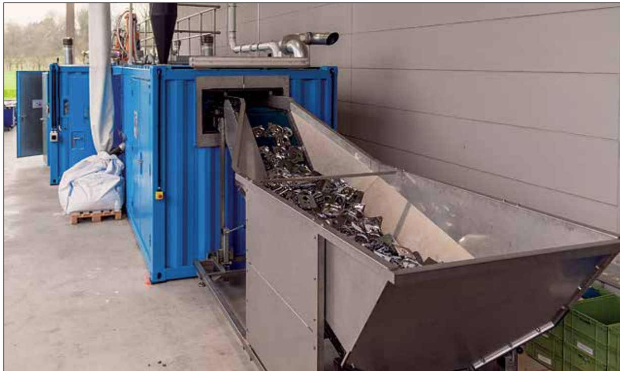
An in-house-designed facility for stripping chrome-plated plastic parts through shockwave treatment, in combination with pre-shredding and magnetic separation, was commissioned at sanitary engineering manufacturer Hansgrohe at the start of the year.
