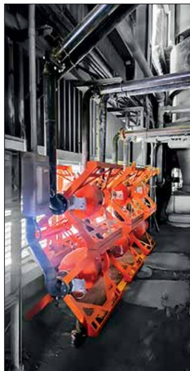
Martin X-Stand set away from the hot wall with pipes running overhead.
