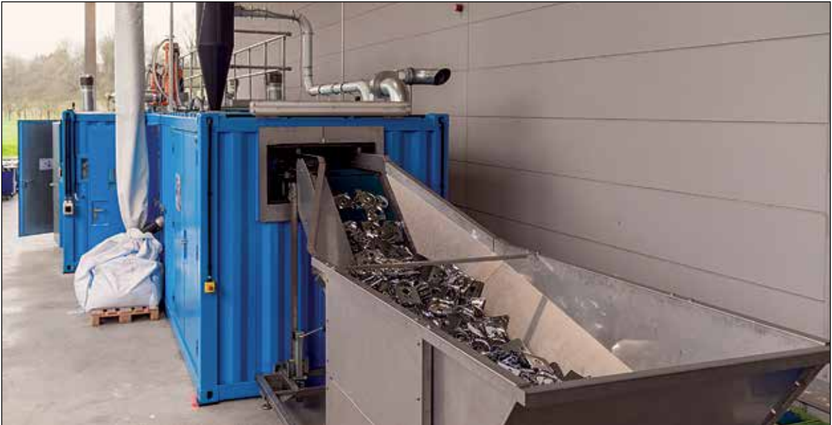
An facility for stripping chrome-plated plastic parts through shockwave treatment, in combination with pre-shredding and magnetic separation, has been commissioned at sanitary engineering manufacturer Hansgrohe (see p9).
