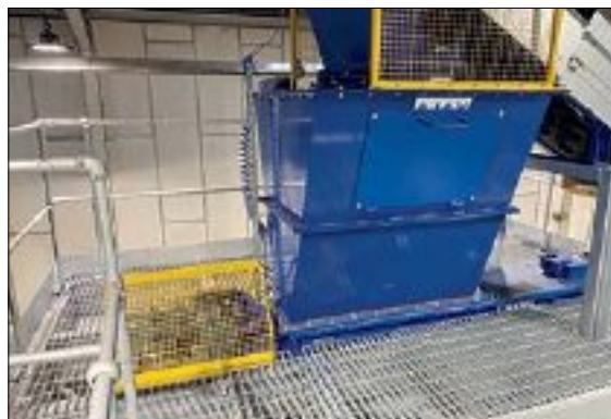
The Ajax Equipment hopper holds approximately 1 ton of iron ore and additives.
