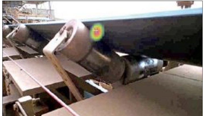
The health of the conveyor belt bearings is critical. Identifying early signs of failure can prevent catastrophic downtime (see p4).
