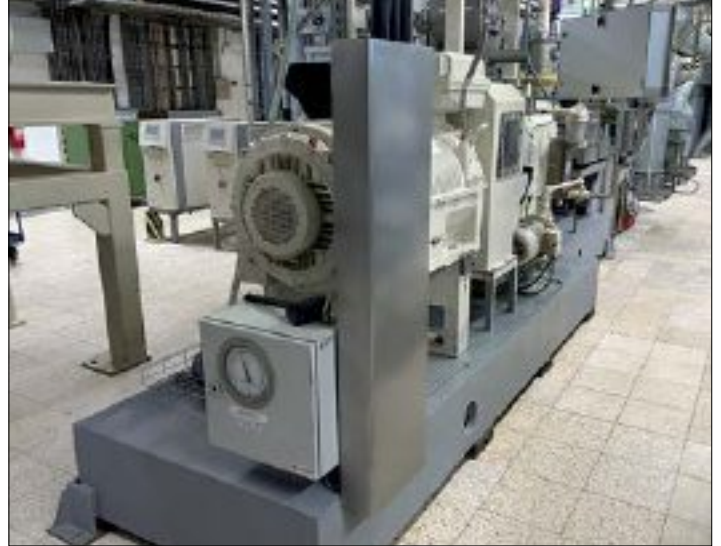
The extruder main drive's control system was swapped out and the ZSK extruder's entire automation was updated.
