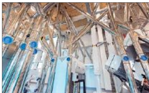
The five-story facility features state-of-the-art infrastructure along with over 70 pieces of equipment from Bühler and its partners.
