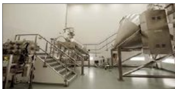
The installation features two Kason MO-B-V Centrifugal Sifters and four Marion Blenders.
