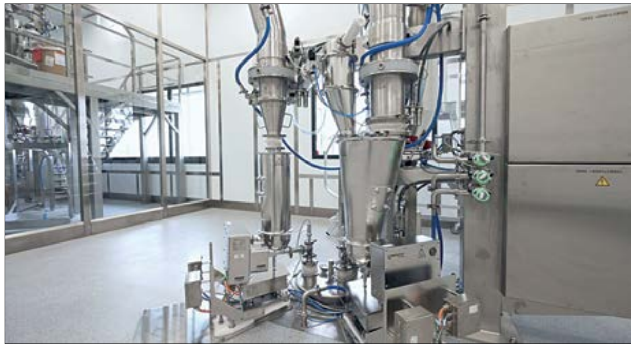
Coperion K-Tron pharmaceutical feeders are an integral part of the Pfizer high containment automated production facility in Germany.
