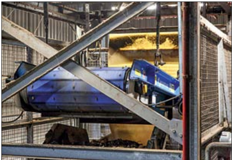
EMAX140 Overband Magnet over the 1.2-metre-wide conveyor.
